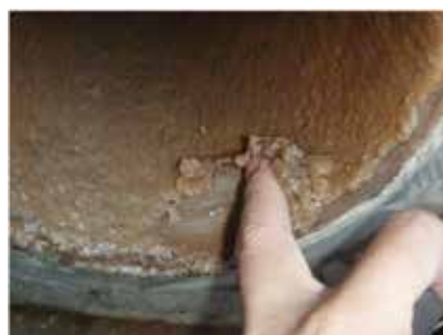
The scale in the circulation pipe can also be easily removed with a finger.
