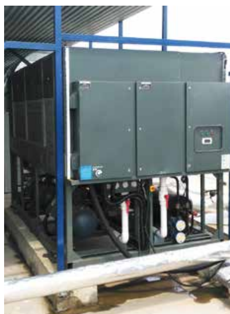
main air-conditioning system
