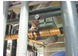
Vulcan S25 impulse cables
