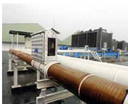
Vulcan S500 was located inside aluminum box and installed on a cooling tower main pipe in Supermal Karawaci.
