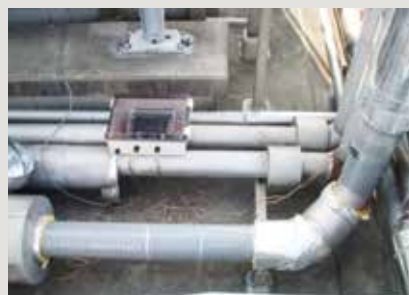
Vulcan S100 installation
