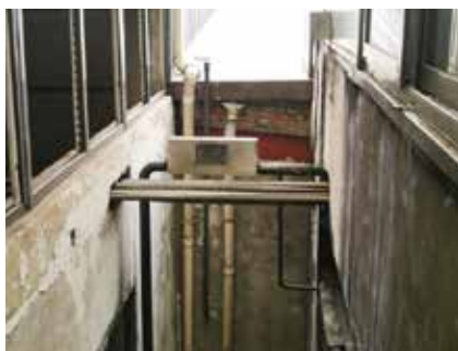
Vulcan S25 outdoor installation
