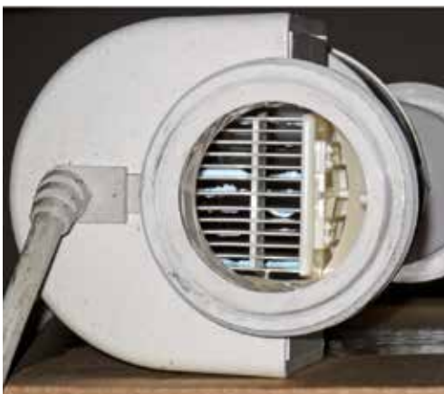
Swimming pool chlorinator in service 30 days before installing Vulcan units
