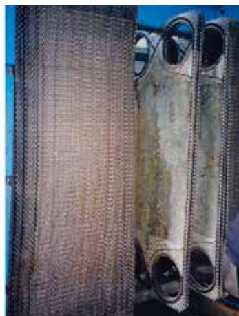
Control of honey comb fill of cooling tower
