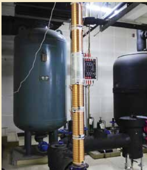
Vulcan S100 installed in the hotel in Beijing, China
