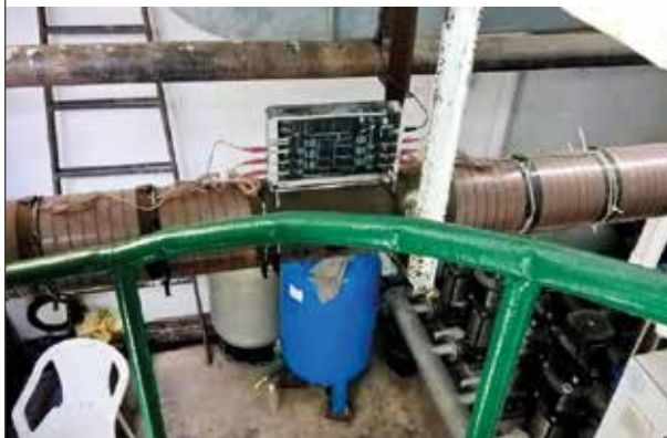
Two Vulcan S100 were installed.
