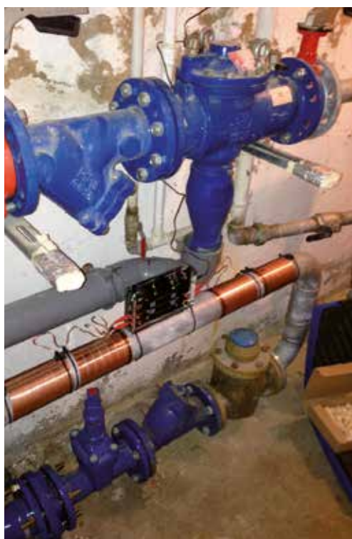
Vulcan S25 installed in the Alcoa Aliminum factory in France
