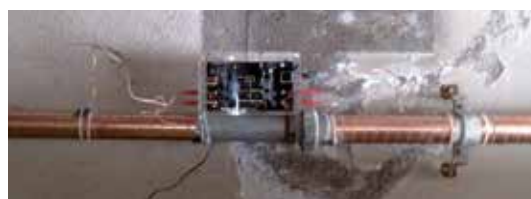
Vulcan S100 installed in the Alcoa Aliminum factory in France
