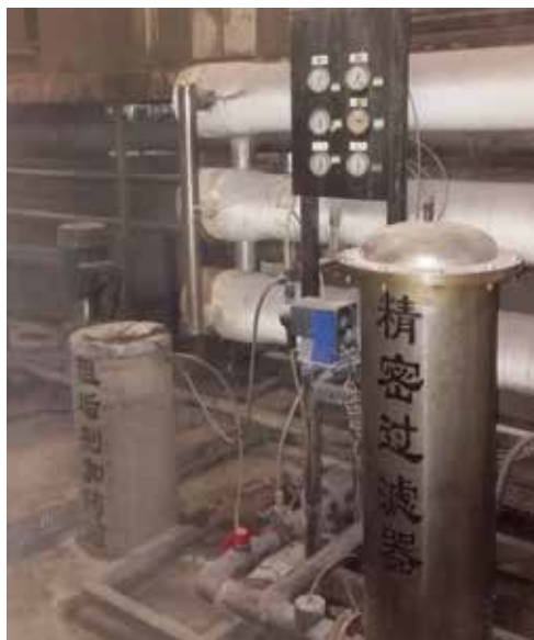
Pure water process equipment.
