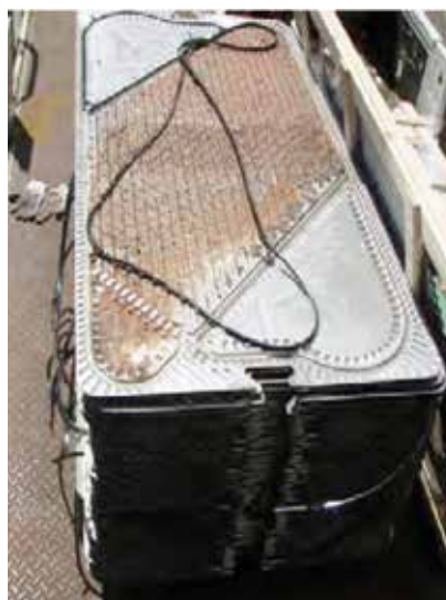
After Vulcan was installed for 9 months: the plate heat exchanger was taken apart for cleaning.
