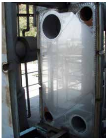
After Vulcan was installed for 9 months: ready open the plate heat exchanger and clean.
