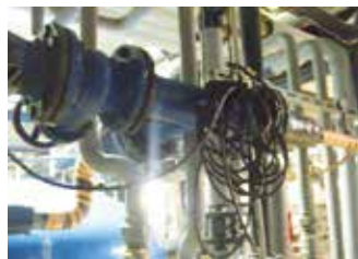
Vulcan S25 impulse cables
