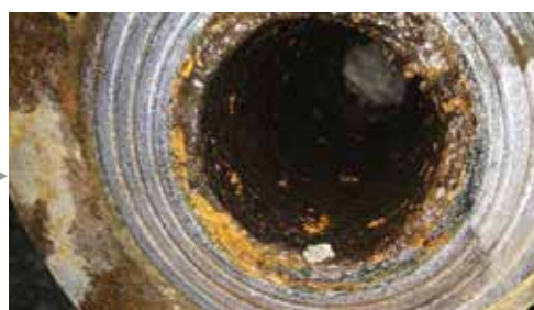
After Vulcan was installed for 3 months, the outer rust had been fallen off completely.
