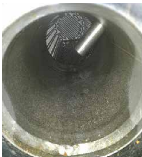
After 3 months – with Vulcan treatment. Up to now the installed pipe line needed no cleaning.
