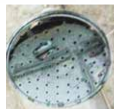
After installing Vulcan for 2 months, the scale of shower head has been reduced.
