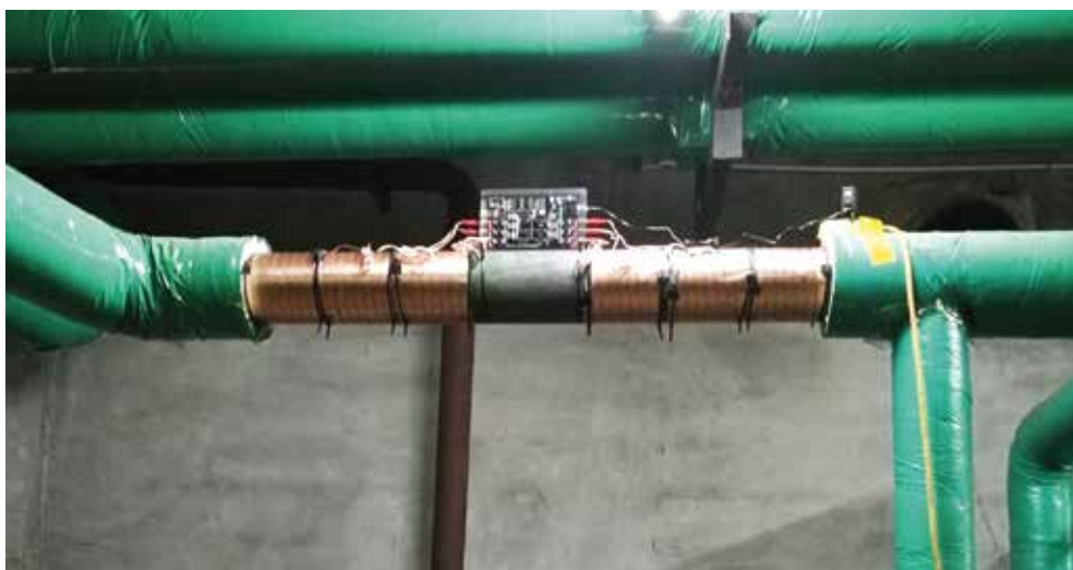
Vulcan S100 was installed on the main circulation water supply, which is from the municipal water.
