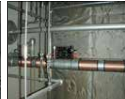
Used for the cooling towers C
