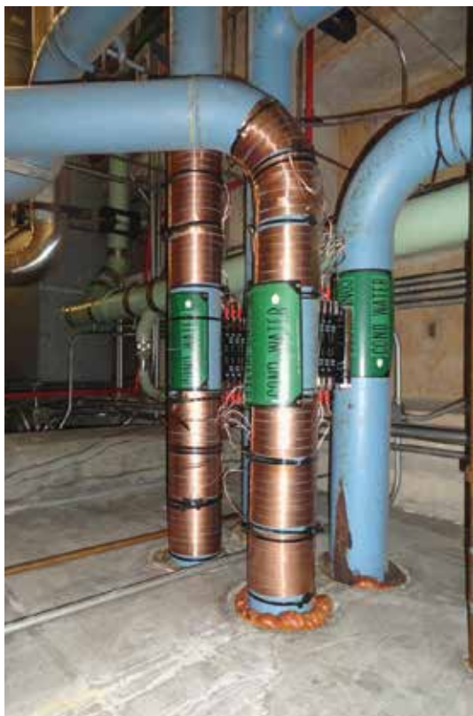
Vulcan S100 units installed on the double chiller
