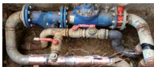
Vulcan S25 installed in the Alcoa Aliminum factory in France
