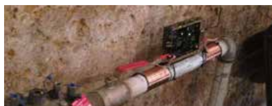
Vulcan S10 installed in the Alcoa Aliminum factory in France
