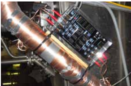
Vulcan S100 unit installed on the produce cleaning system
