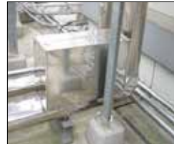
Used for cooling towers A, B and C
