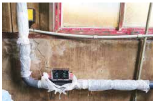
Vulcan S100 in the sewage room for the sludge dewatering machine.
