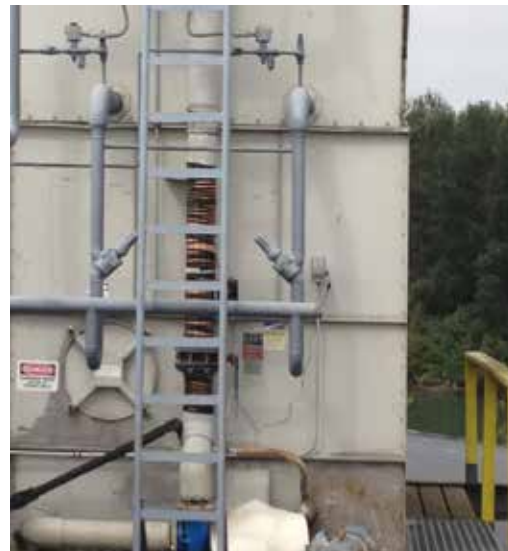
Vulcan S100 installed outside
