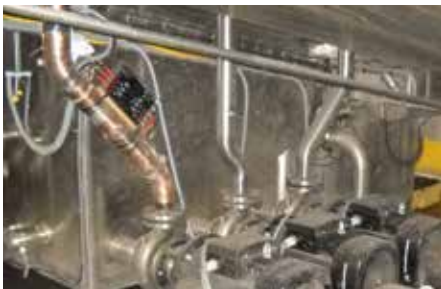
Vulcan S100 units installed on the produce cleaning system
